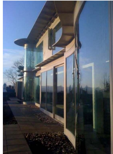
View of the first stages of building to illustrate the quantity of steel involved.
