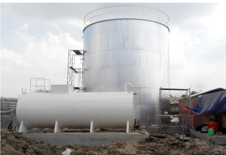
Outside treated tank with Alu topcoat
