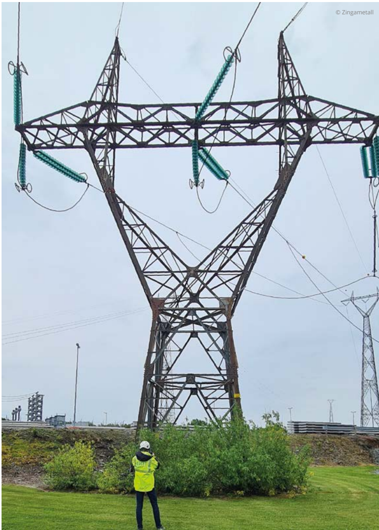
Figure 6 - A typical Norwegian pylon design.
