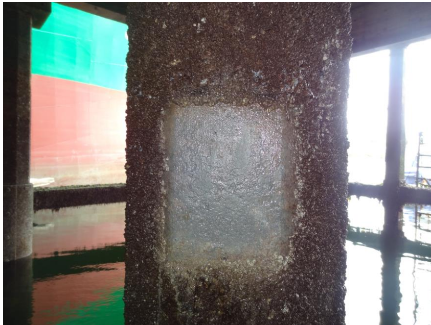
June 2014: Barnacles removed by UHP @ 2700 bars. The Zinga layer is still in perfect condition = no corrosion
