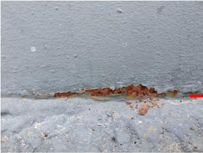
First tank blast-cleaned exhibited corrosion on the bottom 300 mm of the tank-wall above the concrete plinth. Why? The tank was not correctly washed down, leaving abrasive on the steel.
