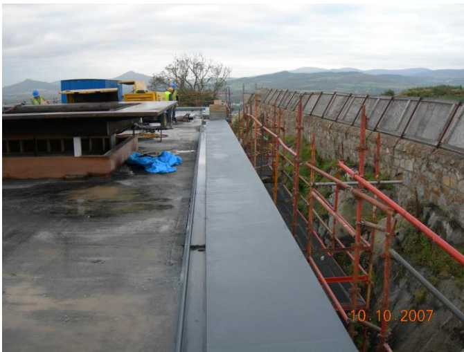
One of the roof edging panels after zingonisation
